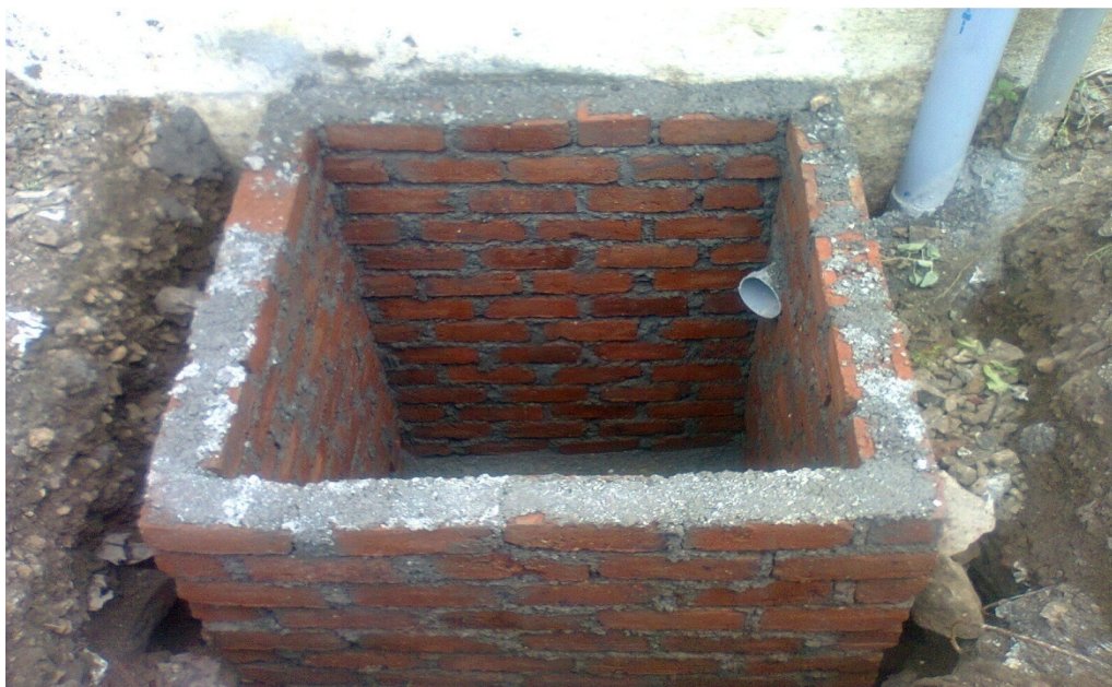
Fig.-2: Underground Collection Tank for collecting Rain Water at one of Site: R.D Pharmacy College, Kada
